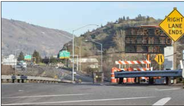
Exit 63, shown, and Exit 64, on Interstate 84 in Hood River will be under construction starting March 2. This is the view from Second Street looking east toward exit 64. Kirby Neumann-Rea photo
