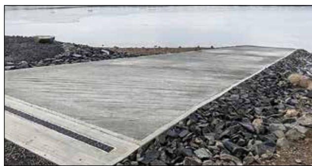
The North Boat Ramp at Pine Hollow Reservoir is now completed, after years of effort. Contributed photos
