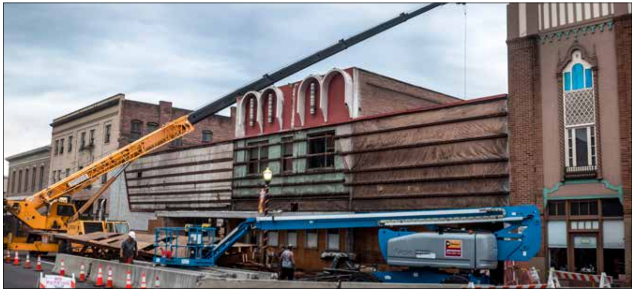
A large crane is used in the removal of the damaged roof from the Recreation Building, where interior beams sag dramatically and banks of ceiling-suspended TVs are askew. A lane of travel remained open for vehicles on Second Street throughout the demolition. Mark B. Gibson/file
