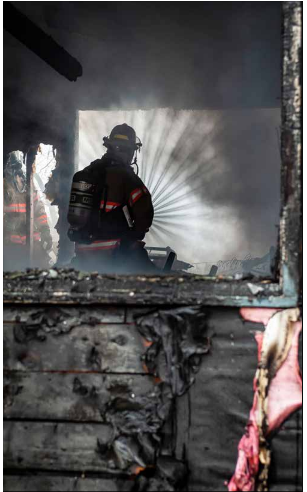
One occupant was burned as they escaped a fire that destroyed much of their home in the 1400 block of Nevada Street in January, 2019. The second occupant was not injured. Mark B. Gibson photo/file
