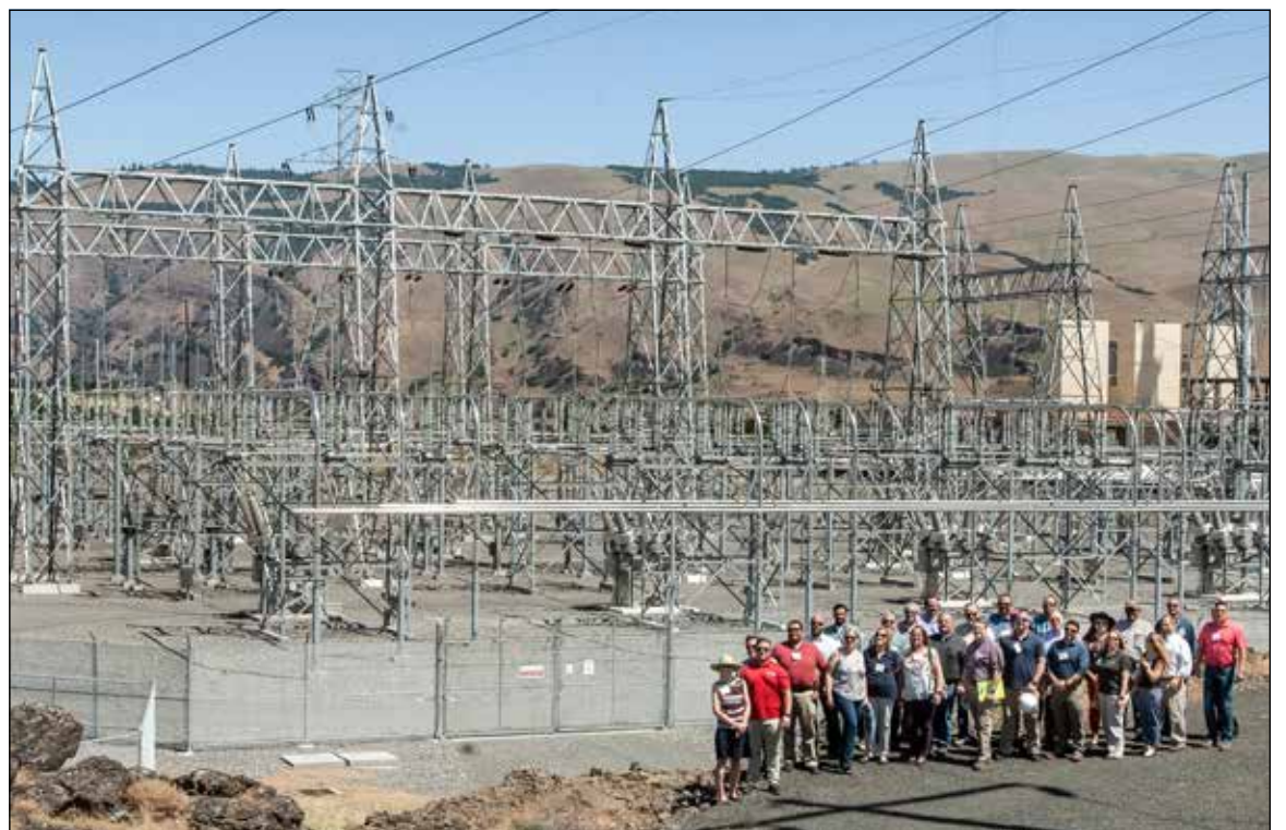
Representatives from throughout the region gather for the dedication in front of the new Quenett Creek Substation in The Dalles for a group photograph. The substation, dedicated in June, increased availability of electrical power throughout the region. Mark B. Gibson photo/file
