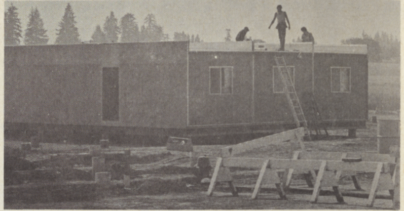
Workmen were kept busy during August putting together the modular units that are used in the temporary student living units.
