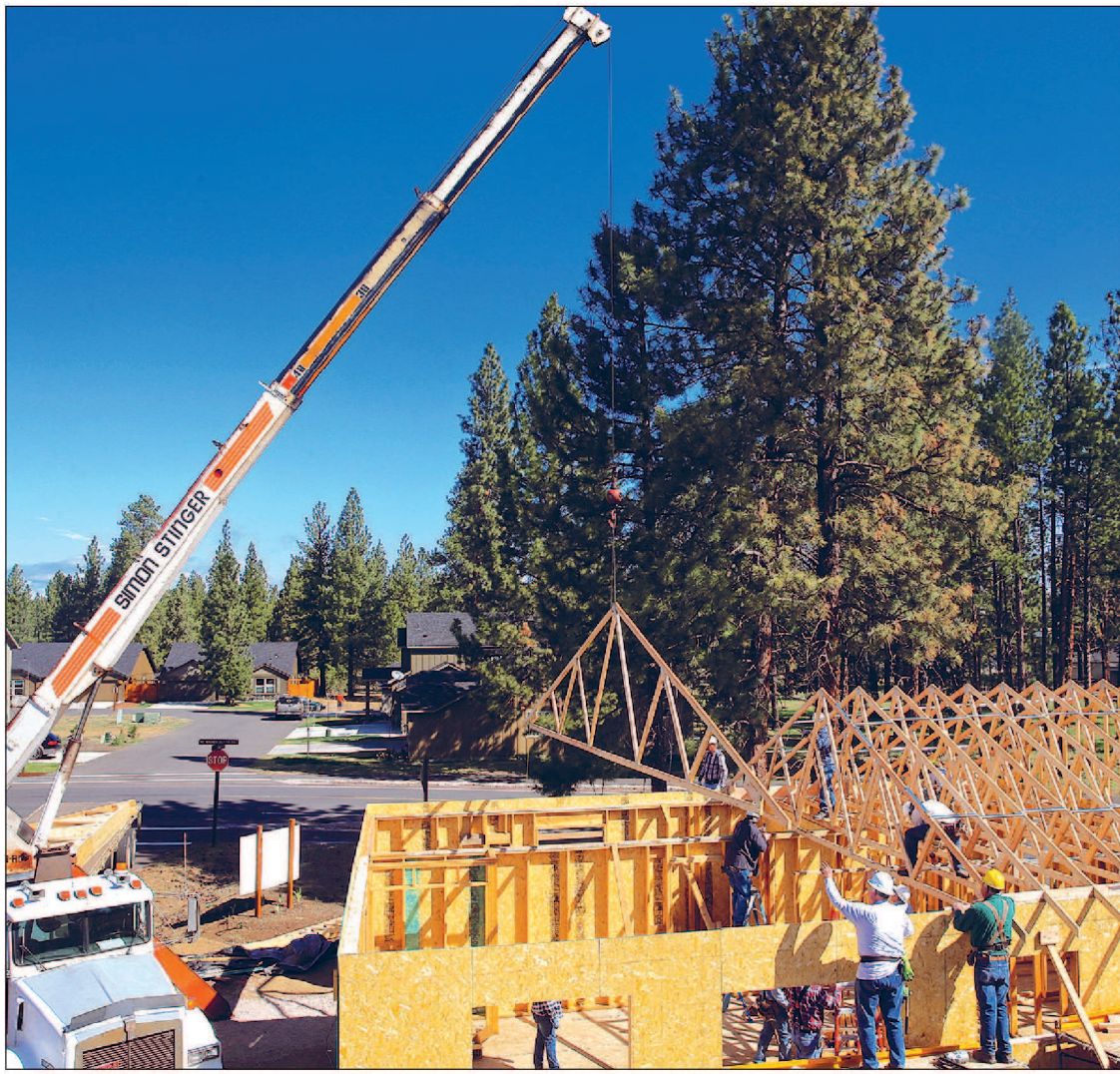
Volunteer work crews set trusses at a new Habitat for Humanity home in Sisters.
