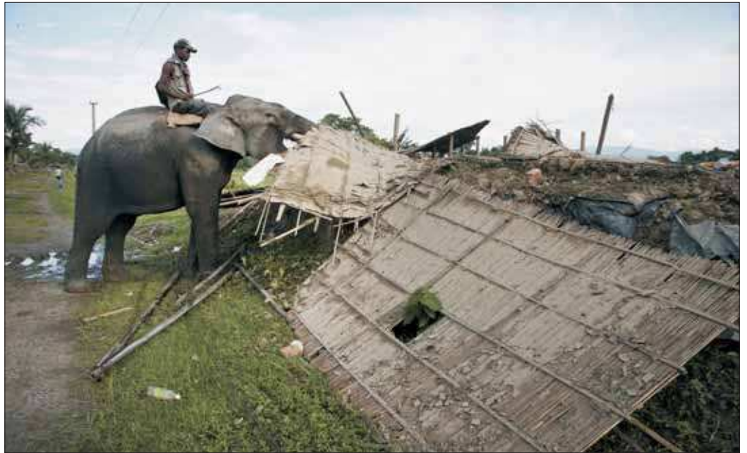
POACHING PREVENTION. A mahout guides a forest department elephant while demolishing a house in Bandardubi village, on the periphery of the Kaziranga National Park in northeastern Assam state, India. Authorities ordered the demolition of about 300 houses in three villages to evict people living on the periphery of the rhino sanctuary to stop rampant poaching of the rare animal, a top police official said. Two people were killed and several others were injured when villagers clashed with police while protesting the demolition of their homes. (AP Photo/Anupam Nath)
