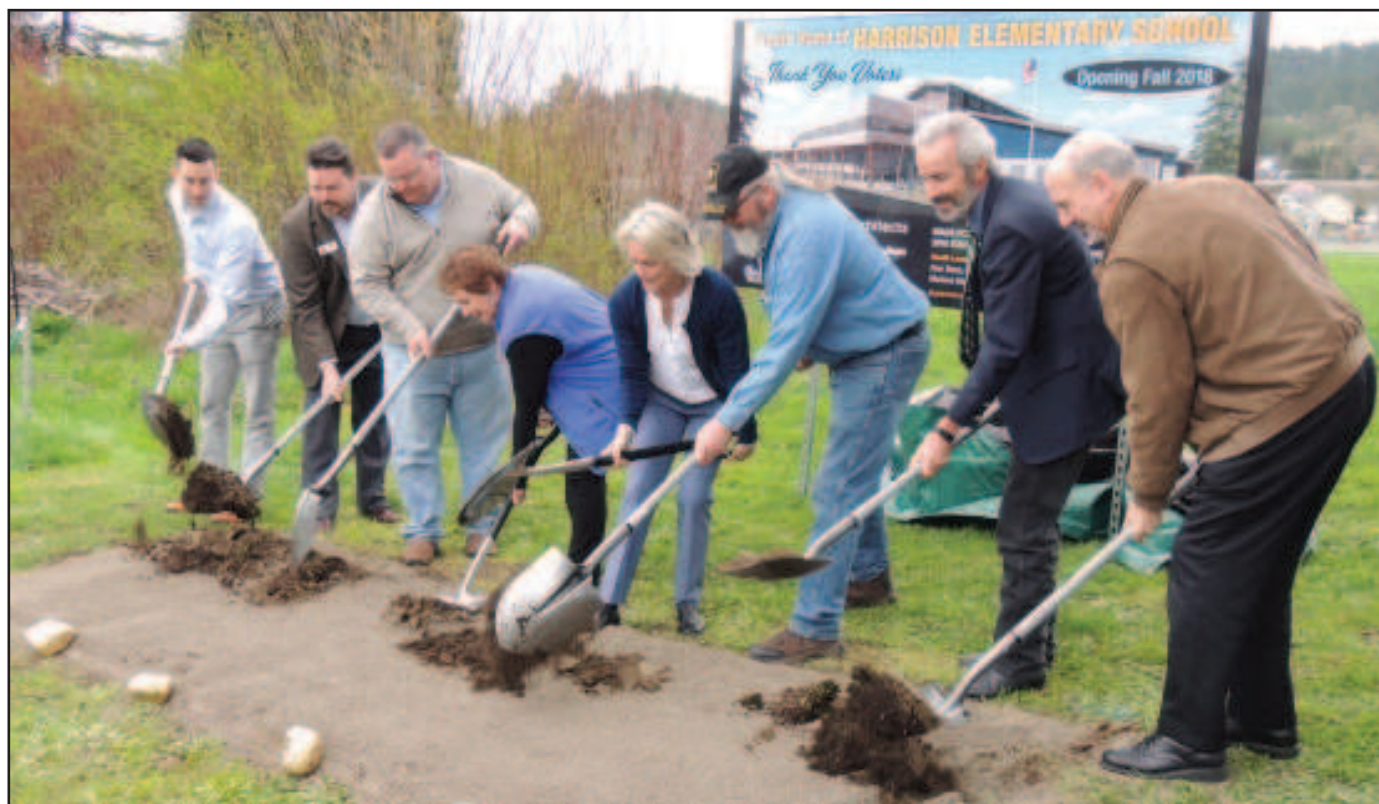
South Lane School District Superintendent Krista Parent joined Cottage Grove Mayor Jeff Gowing, Senator Floyd Prozanski, chamber director Travis Palmer, commissioner Faye Stewart and other local officials to break ground on the new Harrison Elementary School on Thursday, March 23.
