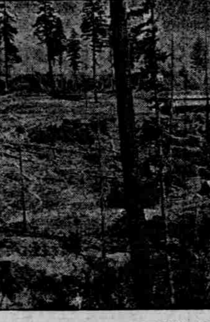
AT THIS POINT NORTHWESTERN ELECTRIC COMPANY IS BUILDING DAM TO GENERATE 20,000 HORSEPOWER.
