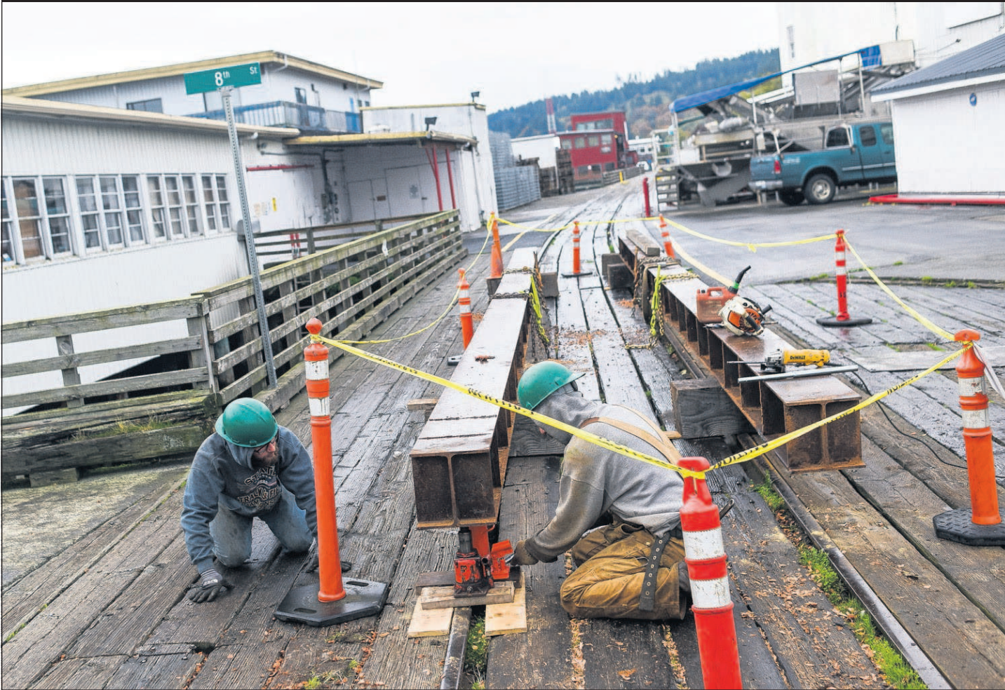
Danny Miller/The Daily Astorian Bergerson Construction Co. employees work on repairs to the rail line on Eighth Street in Astoria Wednesday.
