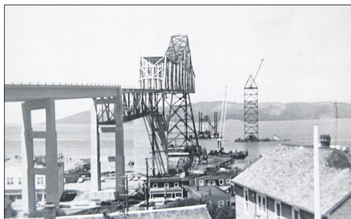
Photo shows Pier 166, built at Tongue Point, being barged into place in preparation for Span 166.
