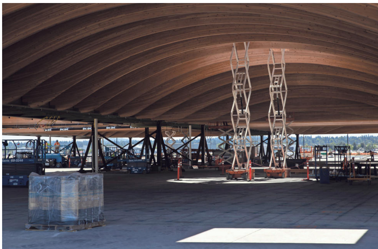
Crews with Hoffman-Skanska work on the new $2 billion remodel of the roof using salvaged wood product from Freres Lumber Co. at Portland International Airport.
