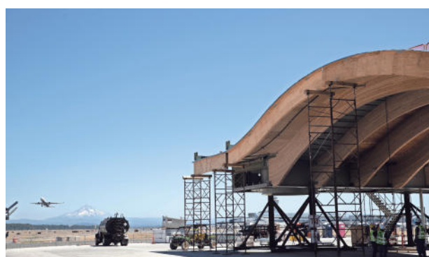
An airplane takes off as crews with Hoffman-Skanska work on the new $2 billion remodel of the roof using salvaged wood product from Freres Lumber Co. at Portland International Airport in Portland, Oregon. BRIAN HAYES / STATESMAN JOURNAL
